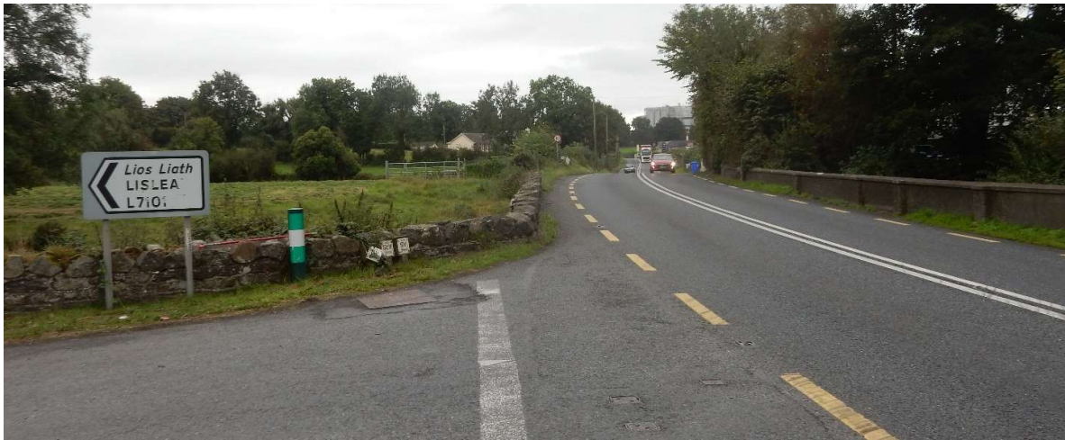
Figure 3-5 Inadequate parapets on river bridge
